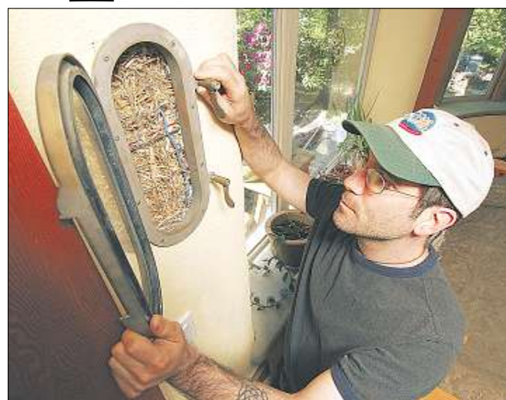
Homeowner Drew Rokeby-Thomas opens the "truth window" to reveal the hemp-bale construction of the home's walls.
